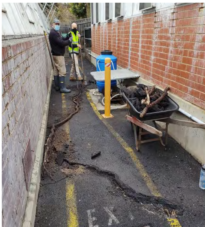
Tree roots in conflict with infrastructure
